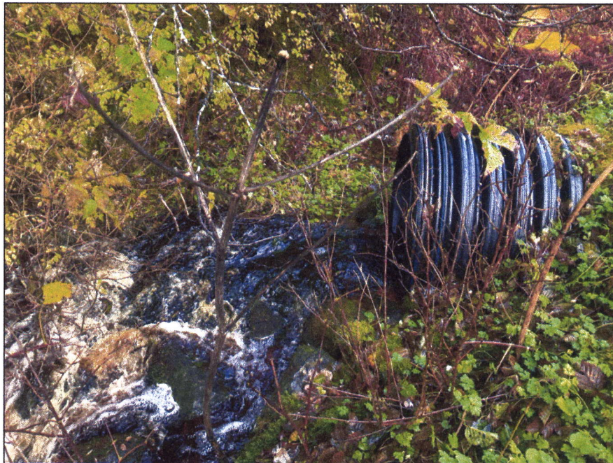
Figure 1.—Outlet of poorly-aligned culvert at waypoint 1018.
