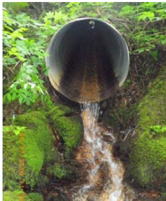
Figure 17: Perched culvert outlet.
