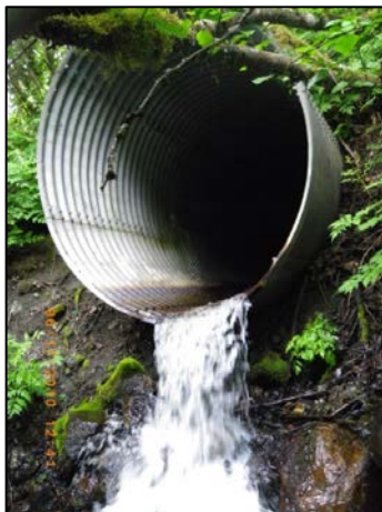
Figure 14: Perched culvert on Falls Creek.
