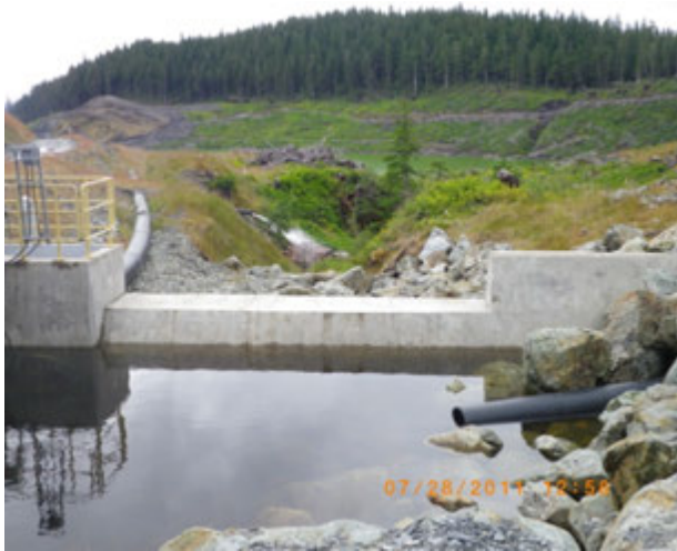
Figure 22. Diversion dam, pipeline, and TTF. Photo by Jackie Timothy.
