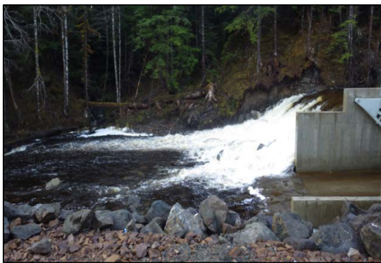
Figure 13.–Gartina Creek overtopping the dam after a rain event, November 9, 2016.
