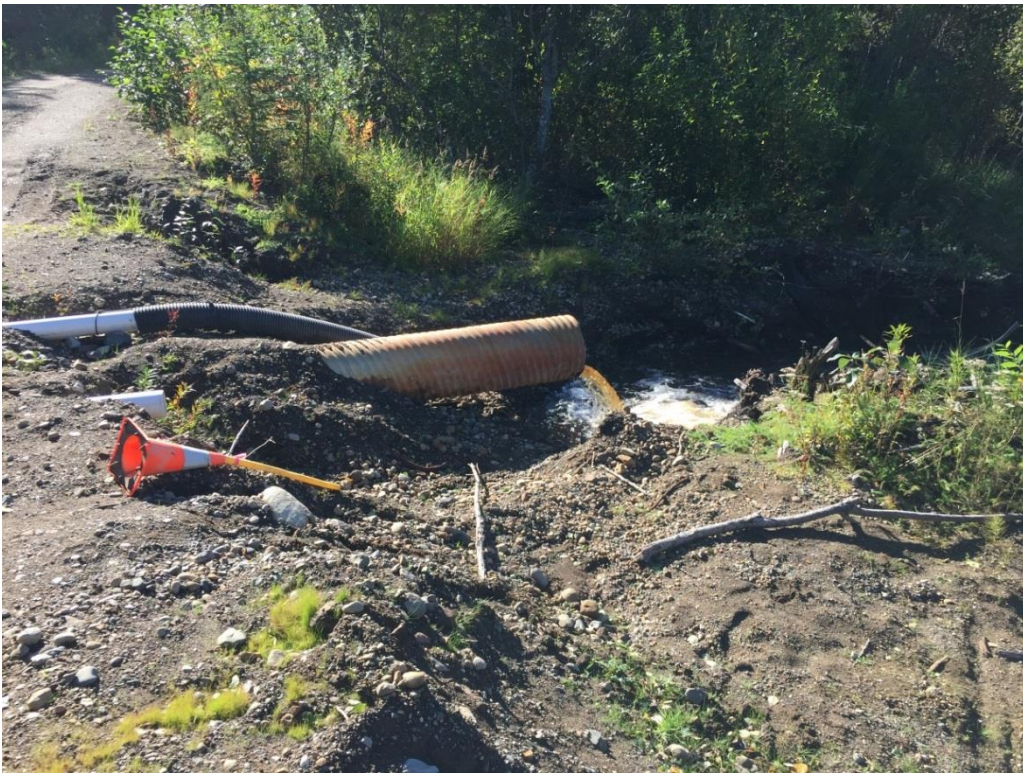
Unpermitted culvert downstream from Site 17-37-1.
