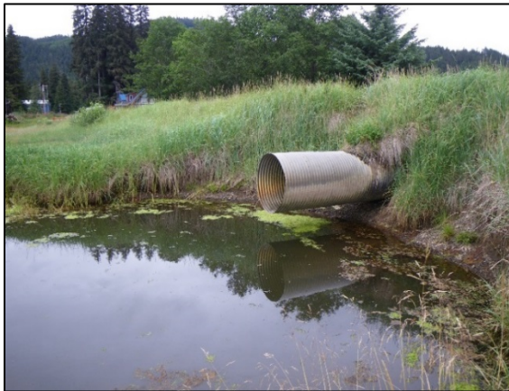
Figure 18.—Perched outlet of Shotter Creek culvert pre-construction, August 2010.
