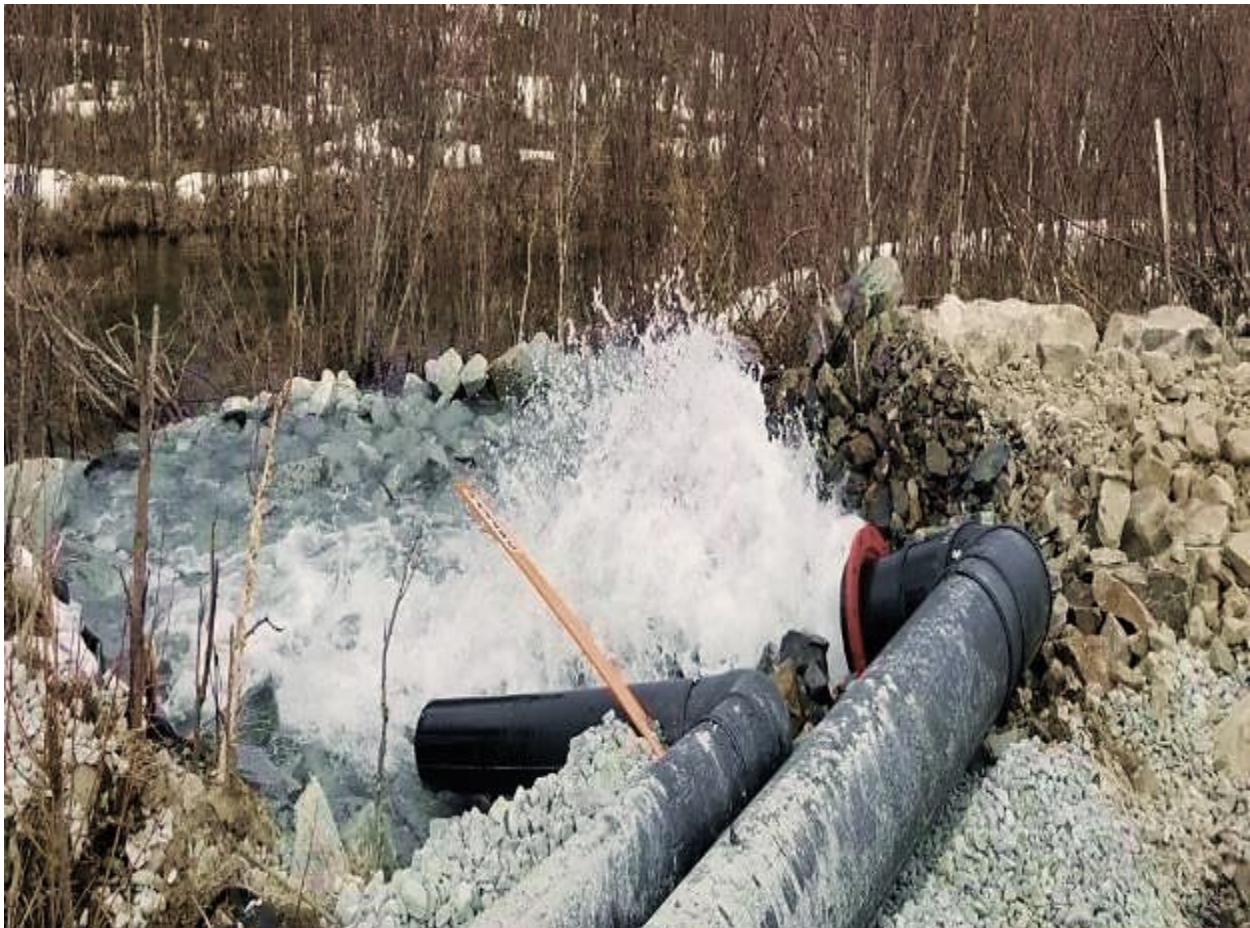
Figure 3. RO Discharge at Outfall 002 on April 10, 2019.
