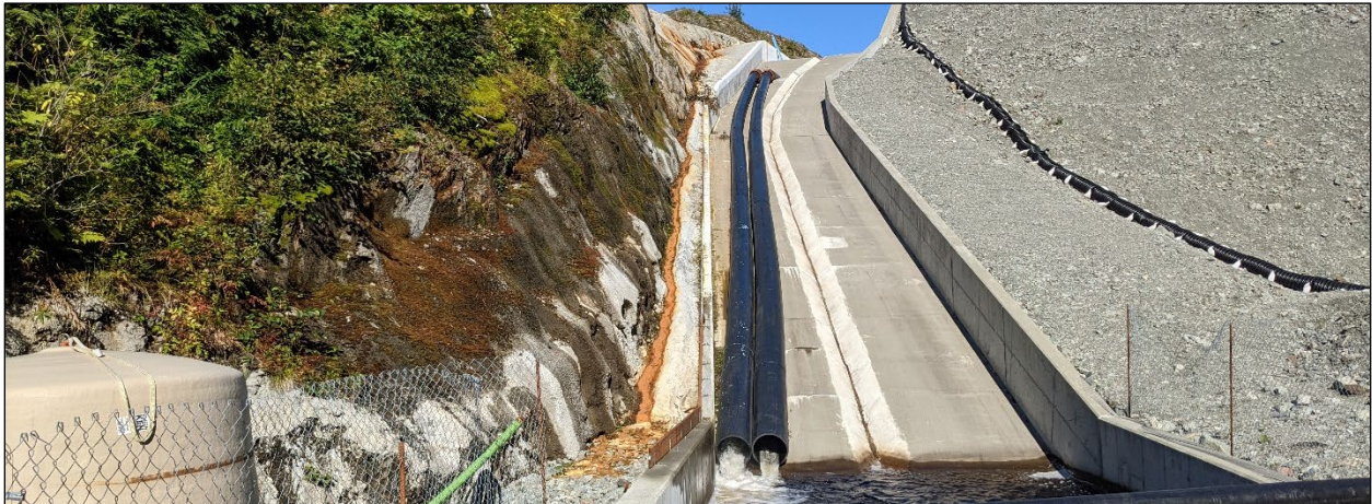
Figure 4.—Tailings Treatment Facility Dam spillway and plunge pool, August 31, 2021. Drainage water from the exposed graphitic phyllite at the west abutment is captured in the seepage collection sump and treated in the Seep Water Treatment Plant.
