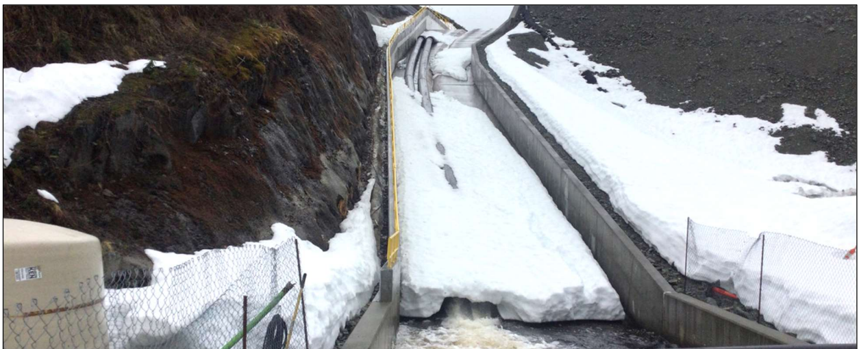
Figure 4.—Tailings treatment facility dam spillway and plunge pool, April 26, 2022. The stage 3 spillway was complete in fall 2021. Drainages from the exposed graphitic phyllite on the west abutment are captured in the seepage collection sump and treated in the TTF seep water treatment plant.
