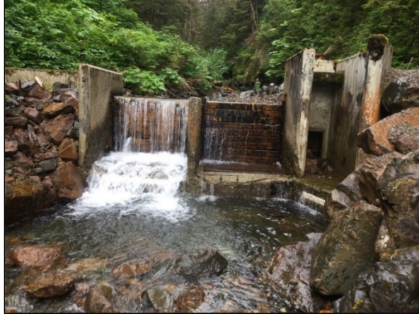
Figure 2.—Existing City water supply intake and location of the proposed hydroelectric facility tailrace, 8/9/2023.
