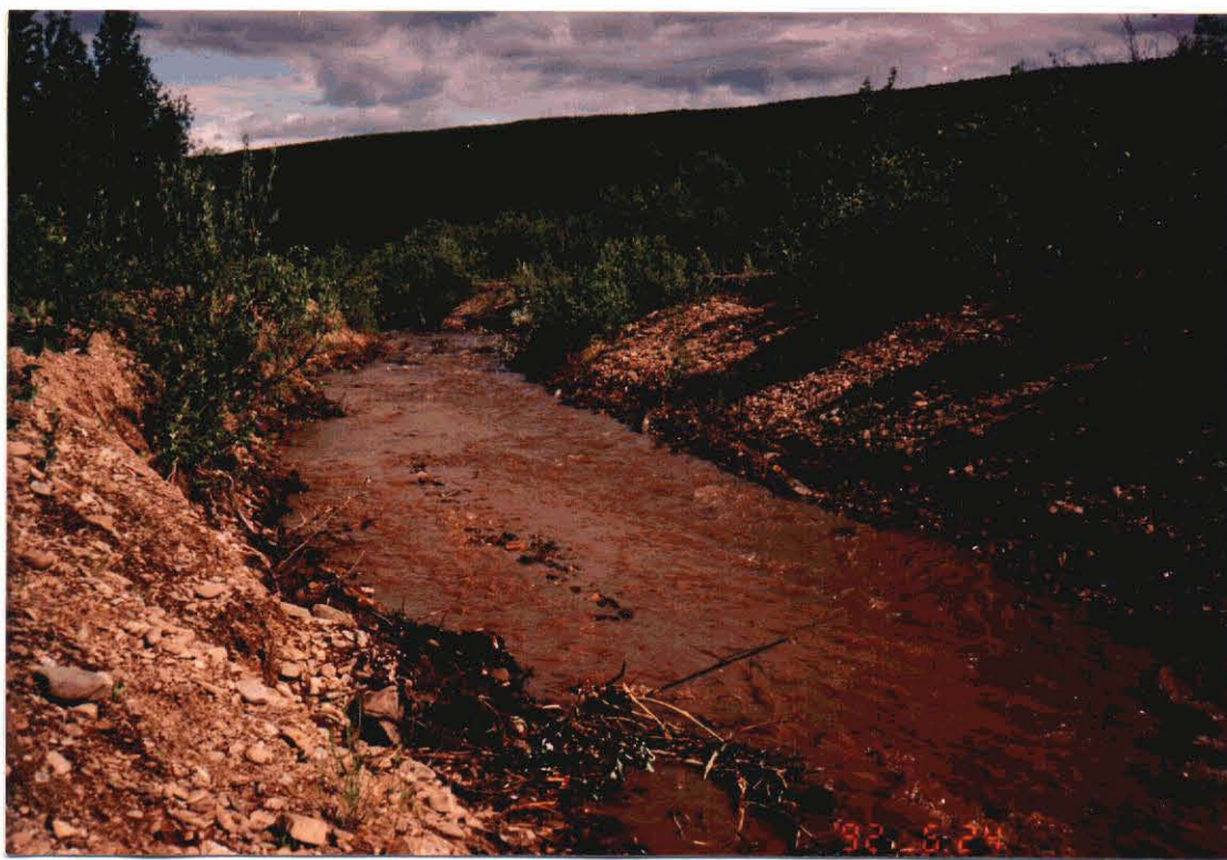
Figure 2. Dozer removing gabion structure from Crooked Creek (top photo) and sample reach #2 following completion of instream work (bottom photo).
