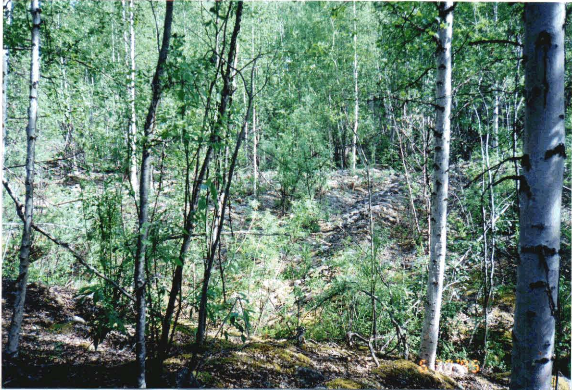
Figure 5. The proposed route of the permanent diversion channel through tailing (top photo) and the constructed permanent channel prior to diversion of water (bottom photo).
